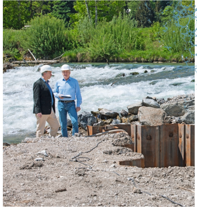
Peter Rutschmann (left) and Albert Sepp aim at reconciling hydropower and environmental protection. For the purpose of advising plant operators and investors on the construction of shaft power plants, they have founded the venture HYDROSHAFT GmbH.
