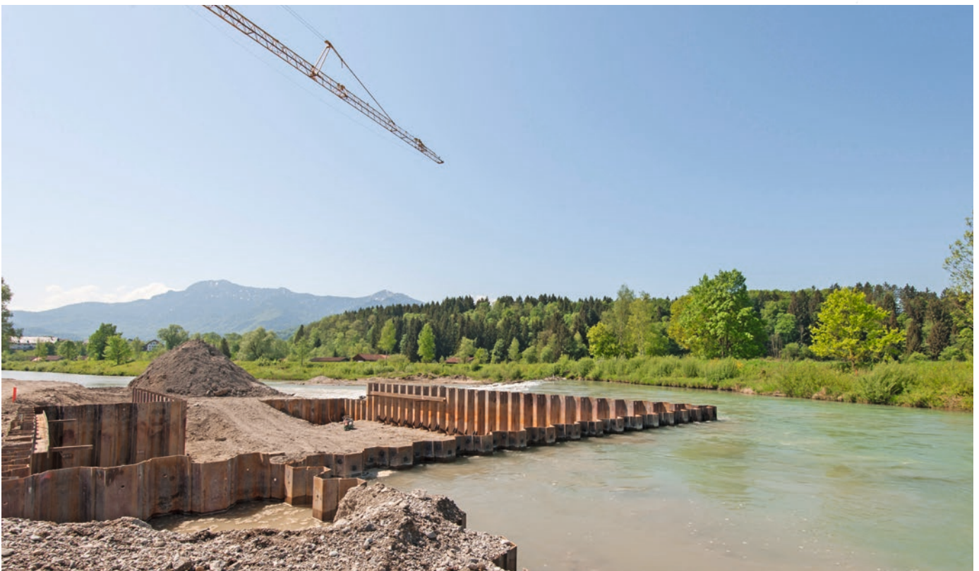
In spring 2018, there is still only the construction pit of the future shaft power plant to be seen. It is scheduled to go on stream at the beginning of 2019.
